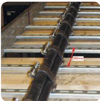
Before short circuit test
