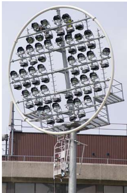
The manrider external-access system at work.
