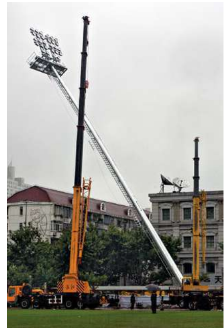
A 40m external-access mast being lifted into position at Shanghai's 80,000 seater stadium.
