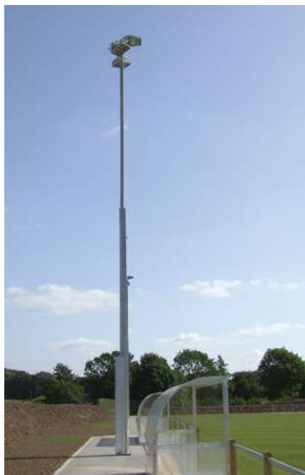
15m telescopic masts at Stone Dominoes Football Club in the UK. The local Planning department permitted a maximum permanent height of 8m.
