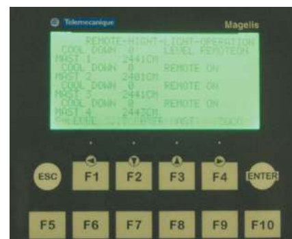
The touch-screen display at Al Shamal stadium in Qatar controls both lighting levels and the telescopic mast system from the main control room.
