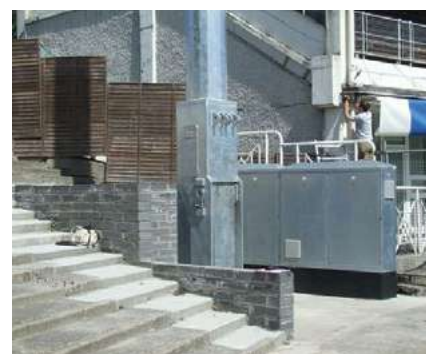
Typical cabinet arrangement for a stadium.
