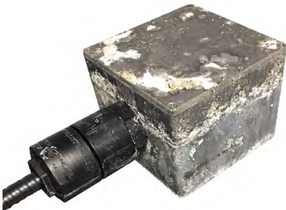
Example of corrosion on Sentinel cable gland
